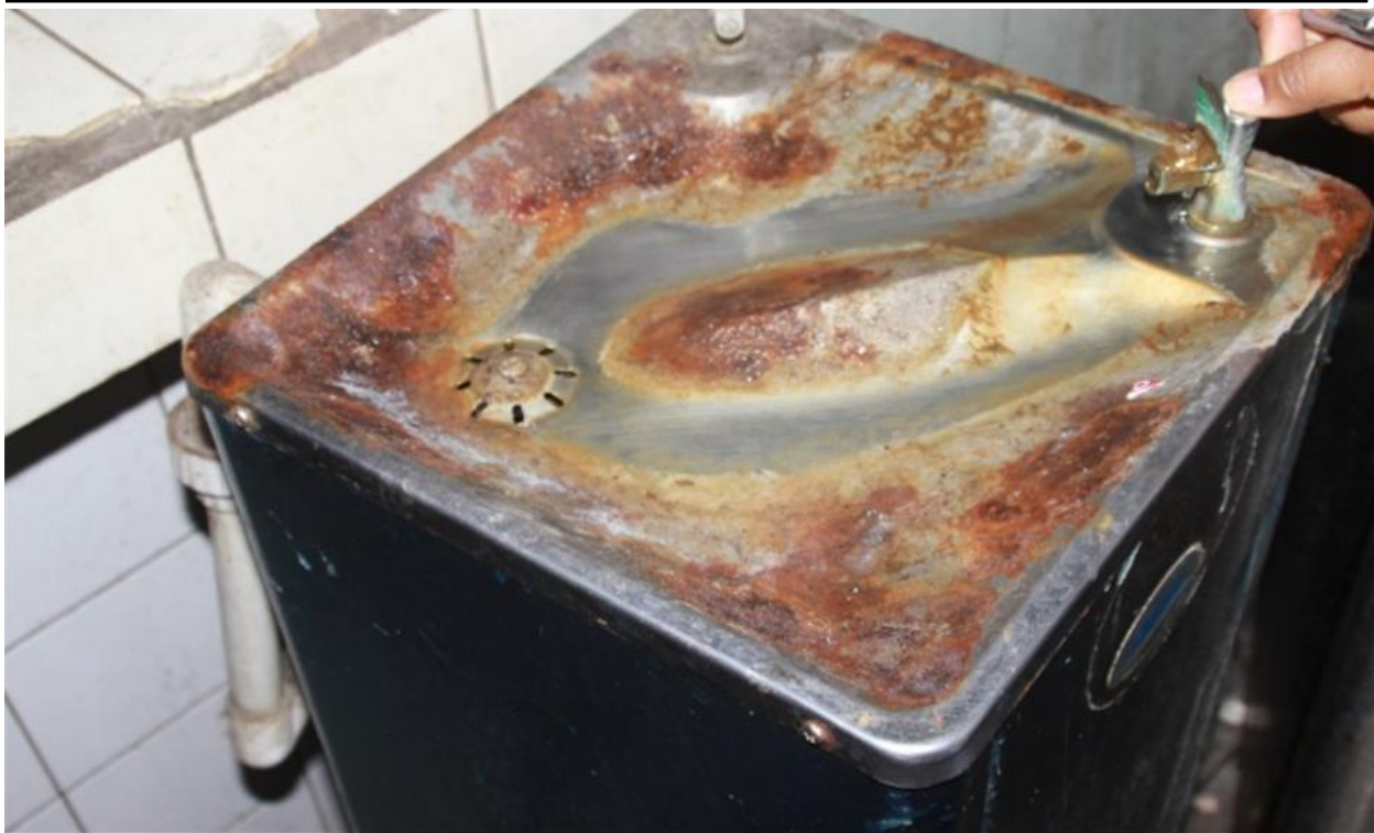
Water fountain at the prison officers' dormitory at the Remand Yard in the Port of Spain Prison
